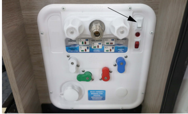
Pump switch -Typical View
