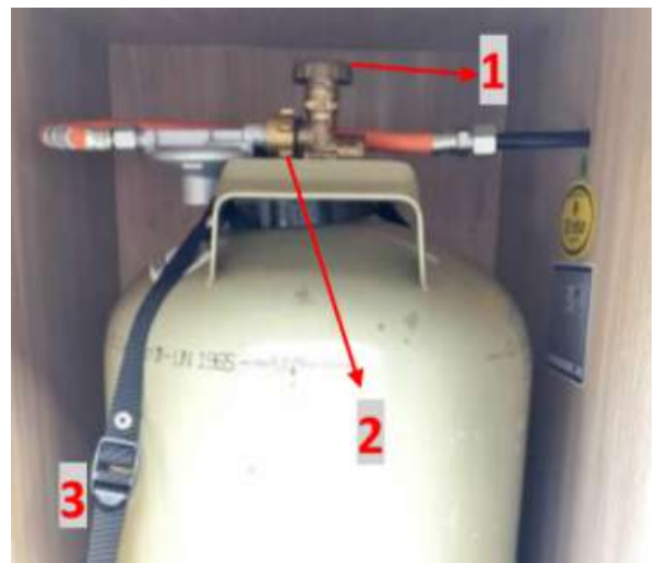
Fig. 4 – Gas bottle installation
