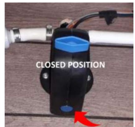
Fig. 6 – Boiler drain valve
