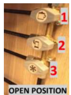
Fig. 5 – Gas shut-off valves
