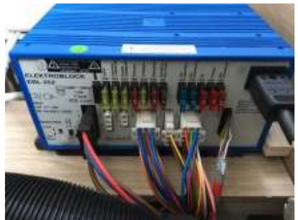
Fig. 2 – Battery charger / Fuse panel
