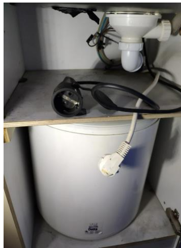
Water Boiler (with its plug disconnected)
